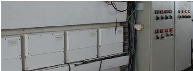
Distributed I/O, installed next to electric boxes
