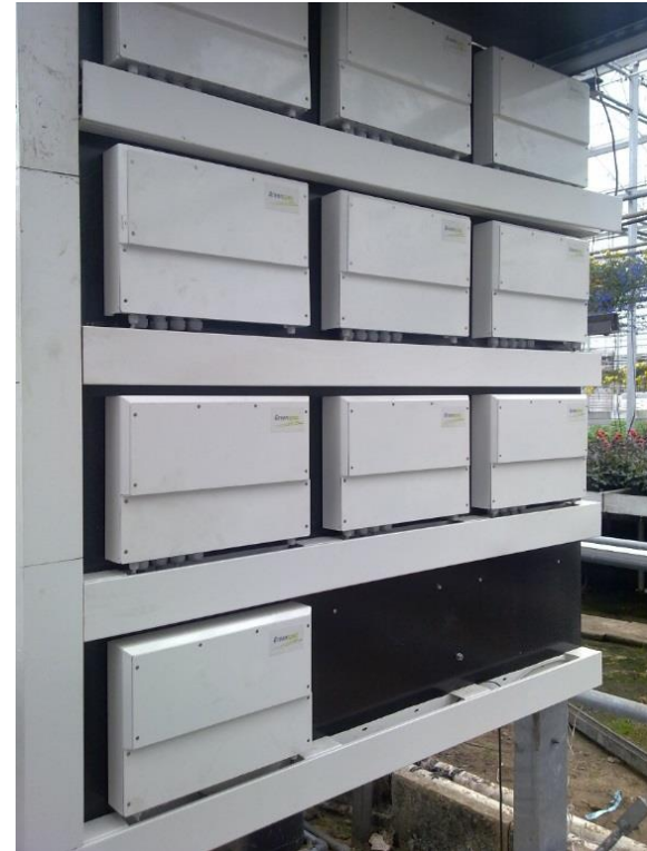
Centralised I/O, installed as replacement of old controllers
